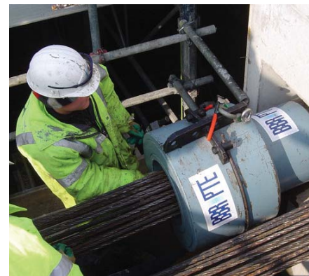
Stressing with a large hydraulic jack and anchoring in a common BBR anchor device.
