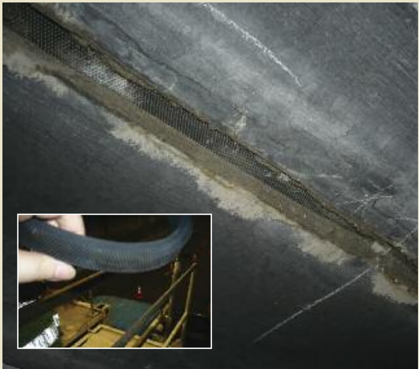
CATHODIC PROTECTION, CENTRAL EXPRESSWAY, SINGAPORE
