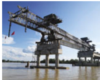
2 The bridge consists of eight spans, each of which is 40.75m long.
