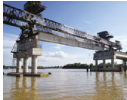
6 The beam launcher was comprised of double trusses and each truss is divided into six equal modules, connected with high tensile bars. It has two main support legs and three auxiliary support legs, attached with hydraulic jacks and a motorized trolley system for level adjustment and transverse shifting of the beam launcher. ●
