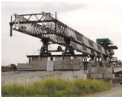
5 The launching cycle is one span per month – including launching of girders, casting diaphragm and deck slab.
