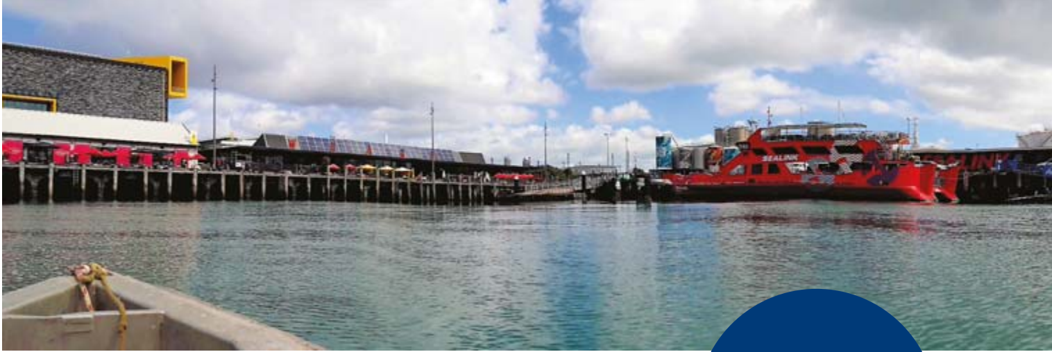
Auckland's Wynyard Wharf is being repaired and upgraded by BBR Contech ahead of the 2021 America's Cup.
