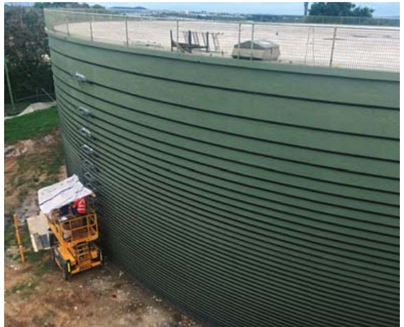
SRG's installation of 43 layers of BBR VT CONA CMB bands around the tank at Mount Pleasant No. 1 Reservoir, means that the town of Mackay's water supply has been ensured for at least another 50 years.
